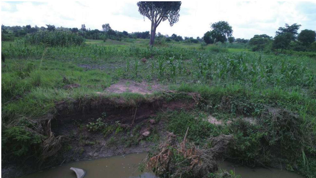
Plate 2: Flooding hot spot at P'Okongo bridge along Tororo-Nagongera-Busolwe road.
